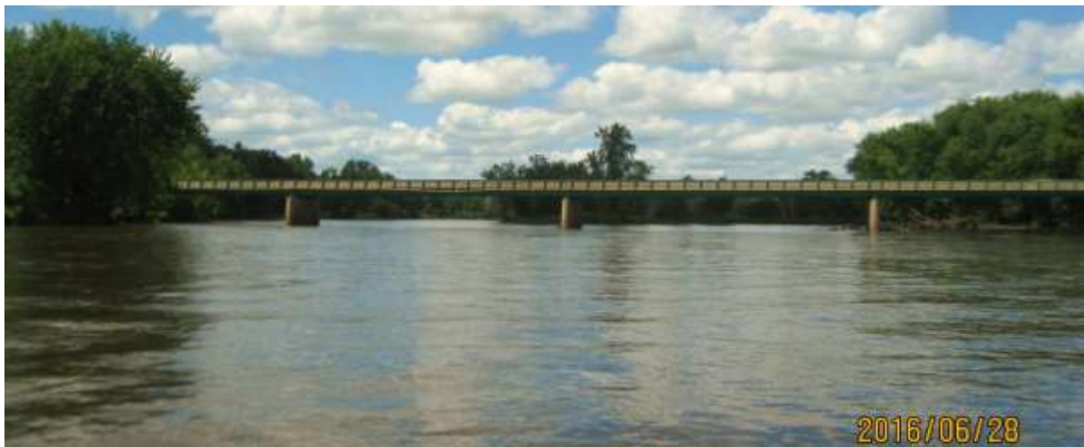
The Cedar Wapsi (C-57) Bridge over the Cedar River viewed from downstream
