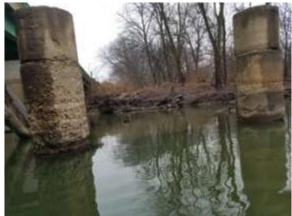
East end of the Cedar Wapsi (C-57) Bridge showing old pilings from a previous bridge _092629
